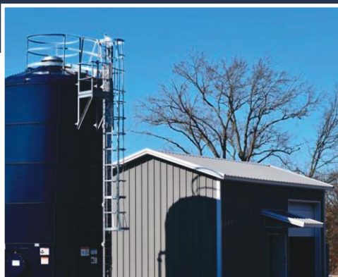
Ferges Water District's new pump station and ground holding tank.
